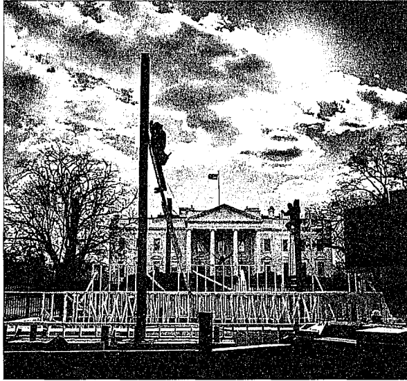
Workers building an inaugural viewing stand in front of the White House are silhouetted against a cold winter sky.
